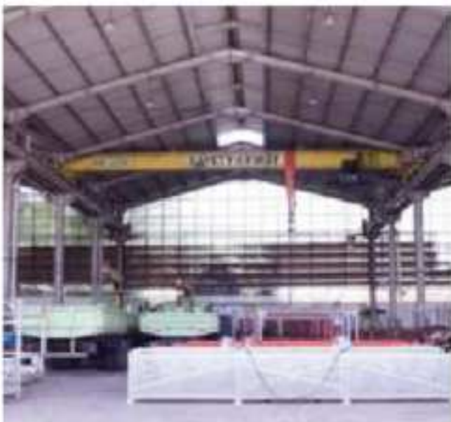
Overhead Crane 10 Ton
